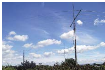
Antennas at GWOGEI: Inverted V for 160m Tx on P80, 204BA 4-el Yagi for 20m and Tennydyne T8 log periodic 10m-20m multi antenna.
